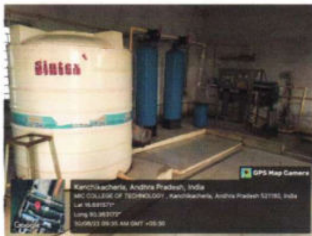
RO Water plant in the campus
